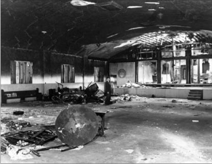
FIGURE 10.3 Arson to cover up theft: fire damage to the San Diego Buddhist Temple. Courtesy of the Japanese American Historical Society of San Diego.
