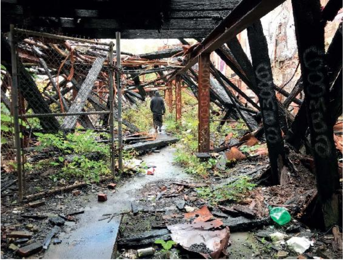
Much of the city's industrial heritage has been consumed by fire.
