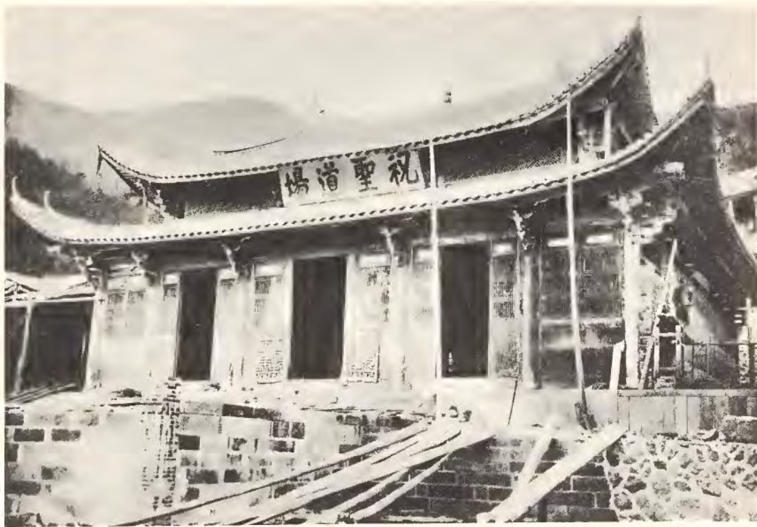
10 A new shrine-hall under construction in 1929 at the Wan-fu Ssu, Fukien, to replace one destroyed by a flood the previous year.
