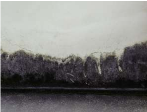
Eikan-dō, detail of wall weathering.
