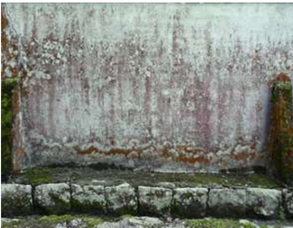
Saishō-in, a subtemple of Nanzen-ji, detail of wall weathering and lichen.
